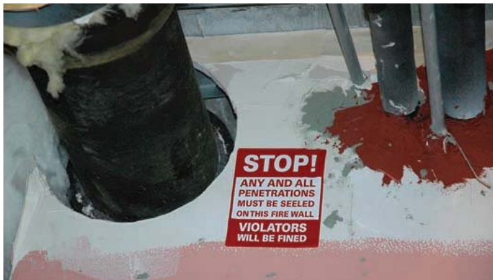
Smoke and fire barrier penetrations are a top cause of Joint Commission citations in hospitals.
